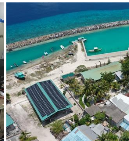
Solar PV at the project site
