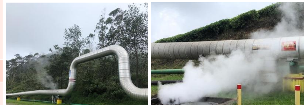
Geothermal steam pipes
