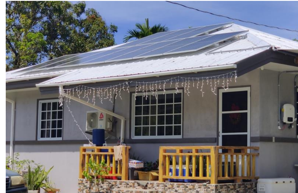
Rooftop solar panels installed under Phase 1 of DRCEF Project.
