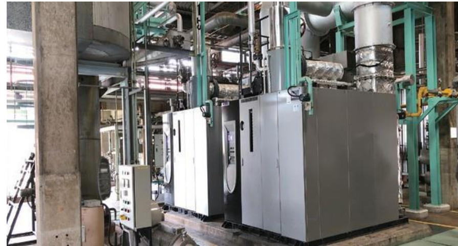
Boiler & Chiller & Solar Power (Thailand)
