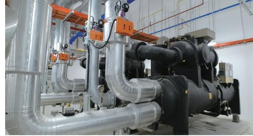
Chiller & LED Lighting (Vietnam)
