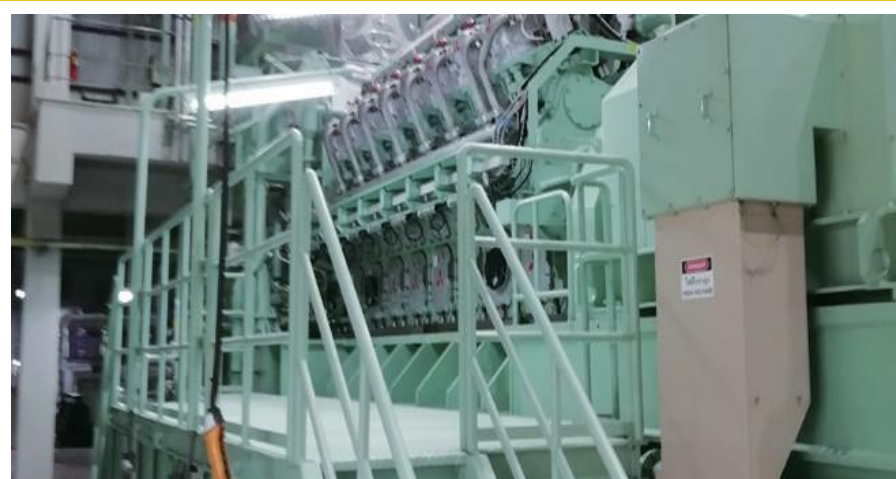
Gas Co-generation & Chiller (Thailand)
