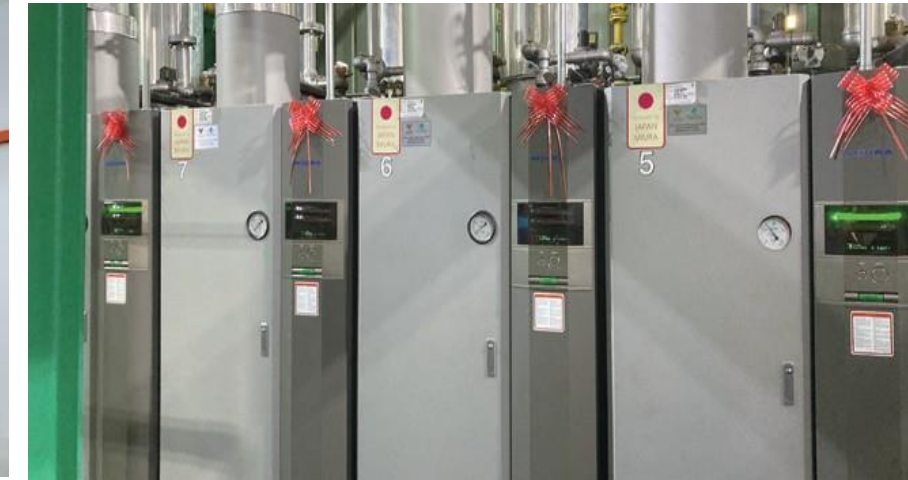
Once-through Boiler (Indonesia)
