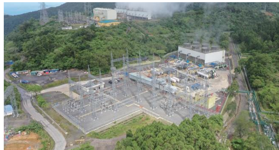
Binary Geothermal Power Plant (Philippines)
