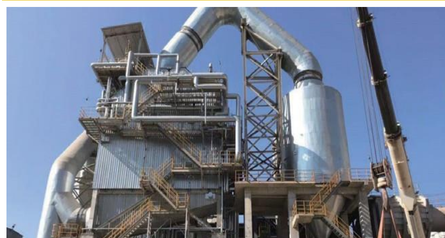
Waste Heat Recovery (Myanmar)
