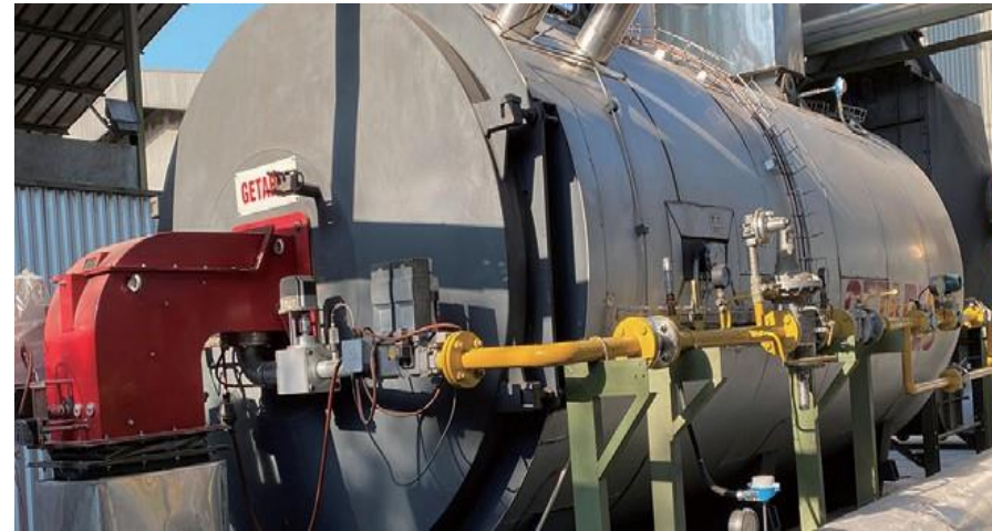
Thermal Oil Heater System (Indonesia)
