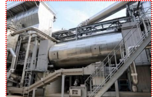
Sewage Sludge Recycling Plant
