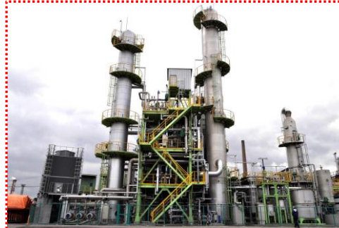
CO2 Capture Plant
