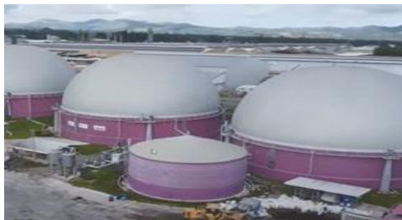
Biogas Power Generation, ITOCHU Corporation, Philippines
