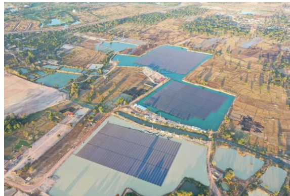
Floating Solar PV, TSB Co., Ltd., Thailand
