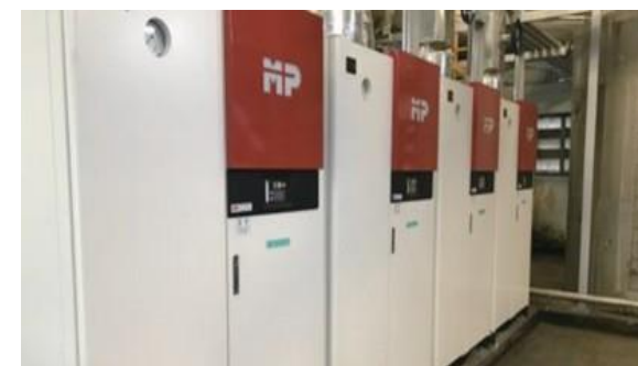
Introduction of High Efficiency Once Through Boiler to Garment Factory, Osaka Gas Co., Ltd., Thailand
