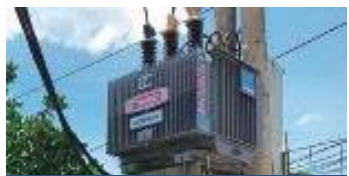
Amorphous transformers in power distribution, Yuko-Keiso, Vietnam
