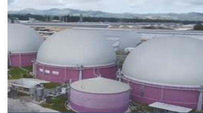
Biogas Power Generation, ITOCHU Corporation, Philippines
