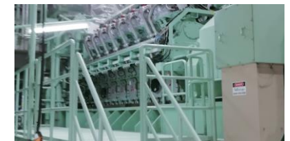
Gas Co-generation System and Absorption Chiller, Kansai Electric Power, Thailand
