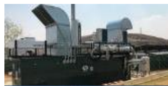
Power Generation with Methane Gas Recovery System, NTTDATA, Mexico
