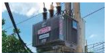
Amorphous transformers in power distribution, Yuko-Keiso, Vietnam
