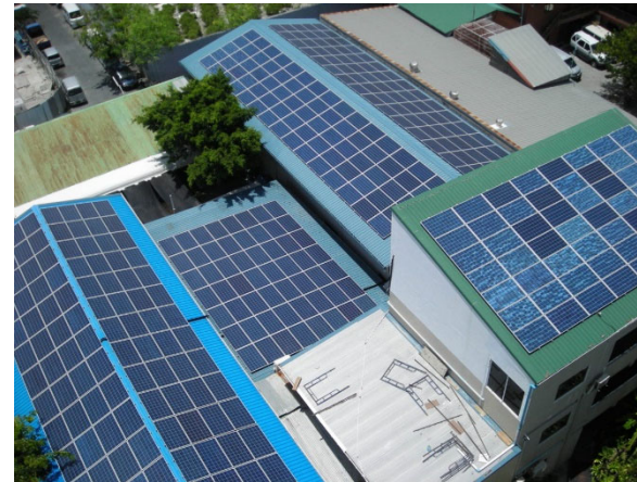
Solar Power on Rooftop of School Building Project (Maldives)
