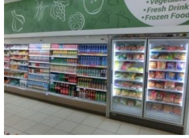
Energy saving at convenience stores, Panasonic, Indonesia
