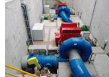
Hydro Power Plant, Chodai Co., Ltd., Philippines
