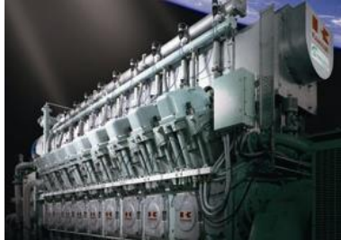
Co-generation system at factory, Toyota, Nippon Steel Engineering, Indonesia, Thai
