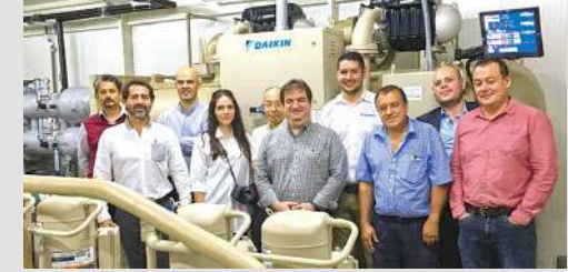
Chiller and Heat Recovery System (Costa Rica)/ NTT Data Institute Consulting Inc.
