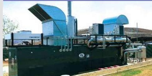
Power Generation with Methane Gas Recovery System (Mexico)/ NTT Data Institute Consulting Inc.
