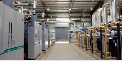
LPG Boilers (Mongolia)/ Saisan Co.,Ltd.
