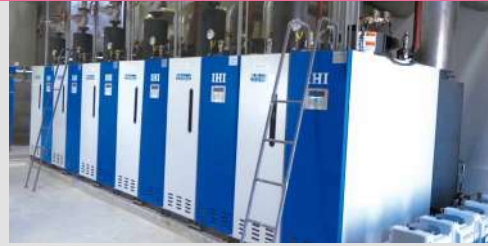
Once-through Boiler (Myanmar)/ Acecook Co., Ltd.
