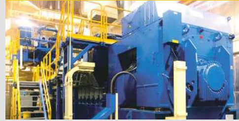
Co-generation Plant (Thailand)/ Nippon Steel Engineering Co., Ltd.
