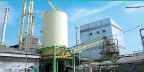
Biomass Boiler (Thailand)/ Fuji Foods Corporation
