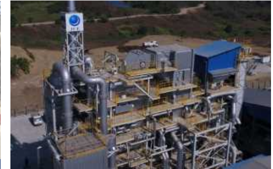
Waste to Energy plant (Myanmar) 4,732 tCO 2 /y. Start operation: Apr. 2017
