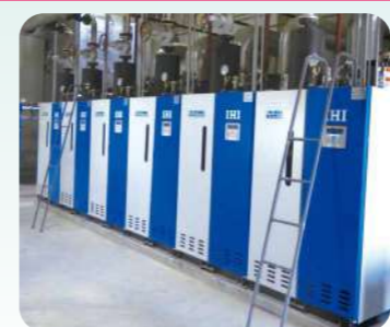
Myanmar / Acecook Co., Ltd. Once-through Boiler in Instant Noodle Factory
