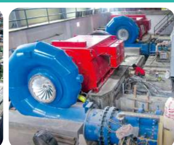
Philippines / Chodai Co., Ltd. Hydro Power Plant
