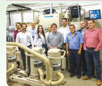
Costa Rica / NTT DATA INSTITUTE OF MANAGEMENT CONSULTING, Inc. Chiller and Heat Recovery System
