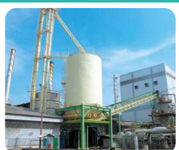
Thailand / Fuji Foods Corporation Biomass Boiler
