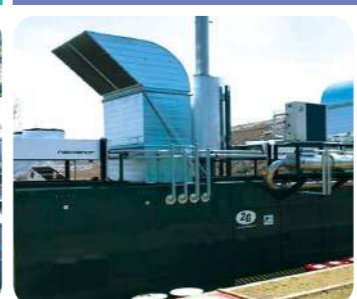
Mexico / NTT DATA INSTITUTE OF MANAGEMENT CONSULTING, Inc. Power Generation with Methane Gas Recovery System
