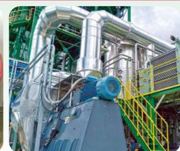
Thailand / KYOWA HAKKO BIO CO., LTD. Refrigerator and Evaporator
