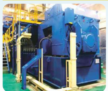
Thailand / NIPPON STEEL ENGINEERING CO., LTD. Co-generation in Motorcycle Factory
