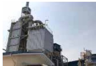
Waste to Energy Plant, JFE engineering, Myanmar
