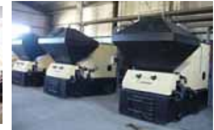
High-efficiency Heat only Boilers, Suuri-Keikaku, Mongolia
