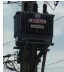
Amorphous transformers in power distribution, Hitachi Materials, Vietnam
