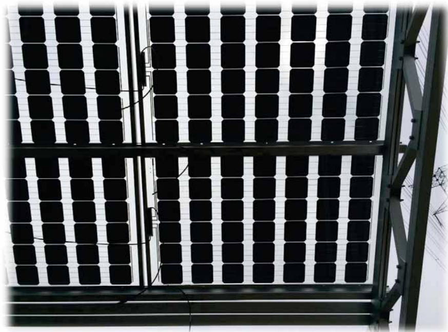
PV modules for greenhouse designed by Farmdo Holdings
