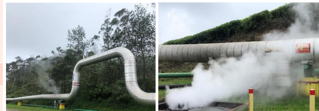
Geothermal steam pipes
