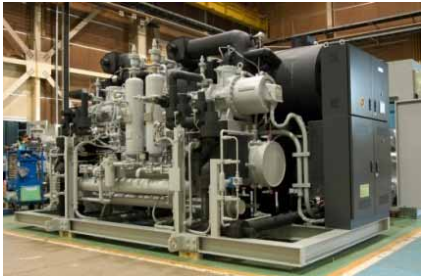
High efficient refrigerator, Mayekawa MFG, Indonesia
