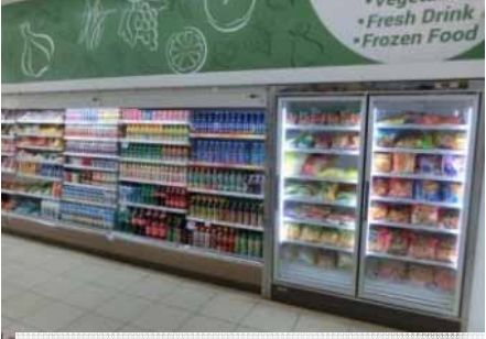
Energy saving at convenience stores, Panasonic, Indonesia
