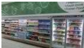
Energy saving at convenience stores, Panasonic, Indonesia
