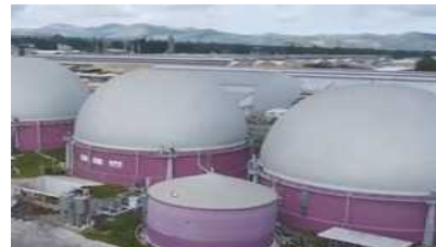
Biogas Power Generation, ITOCHU Corporation, Philippines
