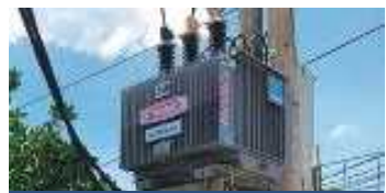
Amorphous transformers in power distribution, Yuko-Keiso, Vietnam
