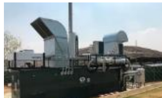
Power Generation with Methane Gas Recovery System, NTTDATA, Mexico
