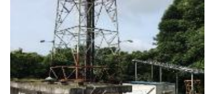
Energy-saving of mobile communications base transceiver stations, KDDI Corp. Indonesia
