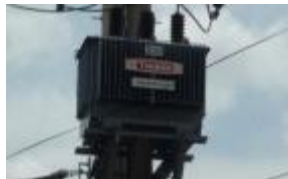
Amorphous transformers in power distribution, Hitachi Materials, Vietnam
