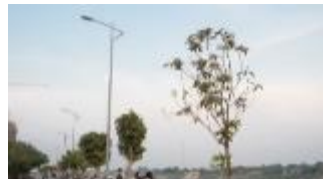
LED street lighting system with wireless network control, MinebeaMitsumi, Cambodia
