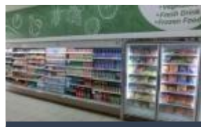
Energy saving at convenience stores, Panasonic, Indonesia
