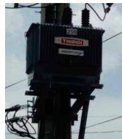
Amorphous transformers in power distribution, Hitachi Materials, Vietnam
