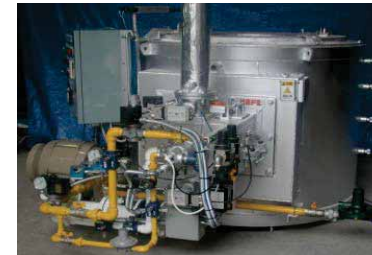
Regenerative Burners in industries, Toyotsu Machinery, Indonesia
